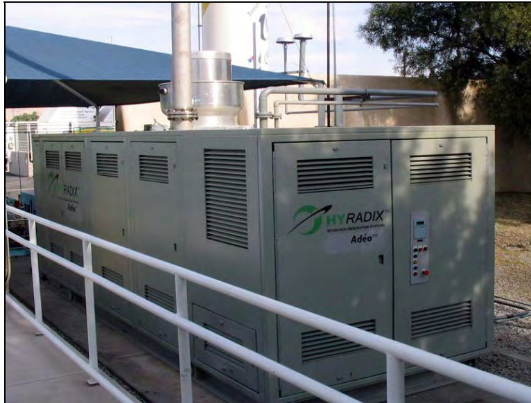
Figure 21. Natural Gas Reformer
