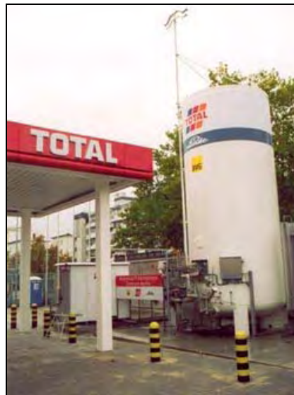
Figure 25. Liquid Hydrogen Storage Station
