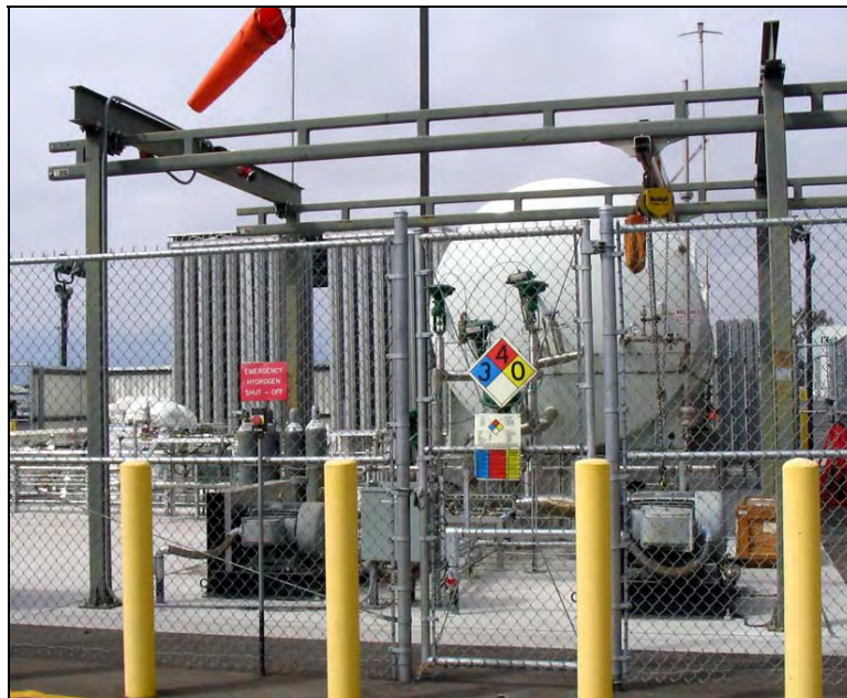
Figure 20. Liquid Hydrogen Storage Tank and Vaporizer
